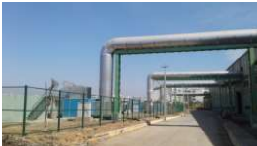
Figure 9. Large biofilter treating exhaust ventilation air 256,000 m 3 /h from 500 tpd integrated solid waste management plant for BBMP, Kudlu, Bengaluru (Licensee: Elixir Enviro Systems Pvt Ltd https://elixirenviro.in/ )
