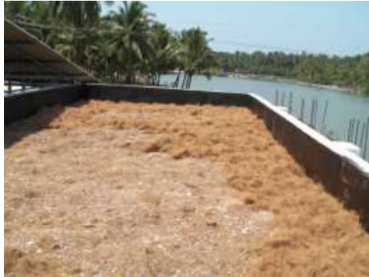
Figure 1. Gas biofilter installed on roof of a fish meal factory. The factory processes low priced sardines and achovy into fish meal protein, a component of animal feed and prawn feed.
