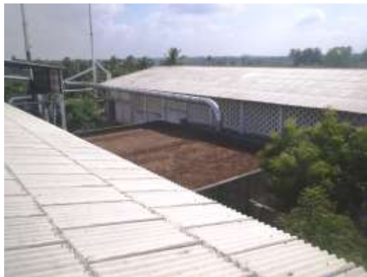
Figure 2. Gas biofilter treating air from two plants making reclaim rubber from scrap tyres. Truck tyres are pulverized and devulcanized to make reclaim rubber sheets, a raw material for tyre manufacture. These factories use chemical devulcanization technology. Without control, odour nuisance can spread for several kilometers.
