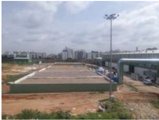
Figure 8. View of very large biofilter installation for municipal solid waste composting plant, Bengaluru (Licensee: Elixir Enviro Systems Pvt Ltd https://elixirenviro.in/ )
