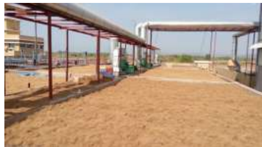
Figure 5. Large gas biofilter (60m x 14.5m x 1.2 m) in 4 independently operable units in fish meal plant at 400 tpd fishmeal plant; February 2016 (Licensee: Elixir Enviro Systems Pvt Ltd https://elixirenviro.in/ )
