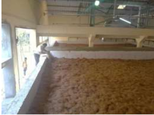
Figure 7. Biofilter for odour from crushed bone processing at ossein unit for gelatin manufacture (Licensee: Elixir Enviro Systems Pvt Ltd https://elixirenviro.in/ )
