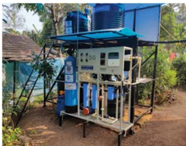
The pilot-scale perchlorate remediation system installed at Kulakkad colony in Keezhmad panchayat, Kerala.
