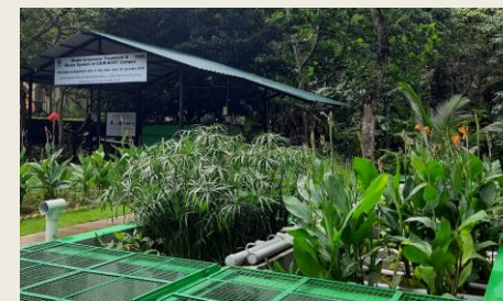
Model Grey water Treatment facility in NIIST campus
